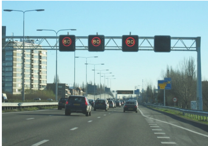
Figure 8: A variable speed limit gantry on the A13 freeway near Overschie, The Netherlands. In this particular case the maximum speed limit is 80 km/h due to environmental reasons, and the limit may drop to 70 km/h or 50 km/h in case of a downstream jam.
